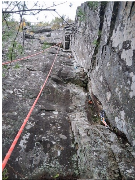
The corner crack of Dodging Bullets .
